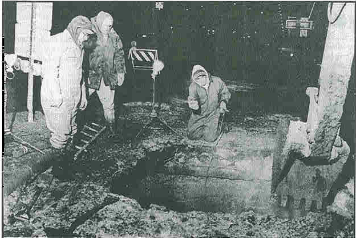
Water main break on Christmas Eve - Temperature -15°. Wind chill -50° (6th Avenue - Holiday Inn)
