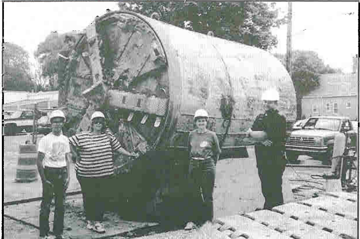
Bob Carlson (right) is showing employees from the Utility's finance division how the auger works for installing the pipe for the tunnel project. (left) Todd Giese, Peggy Walker and Sandi Cisler . - 1993
