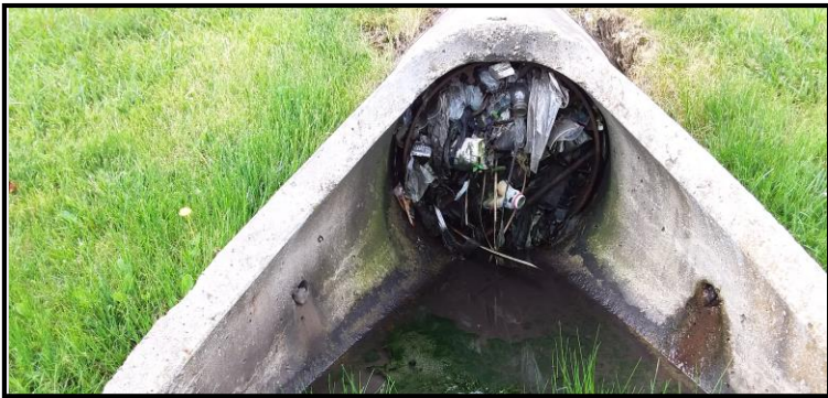
Image 2 A storm sewer pipe clogged with trash. Kenosha 2019
