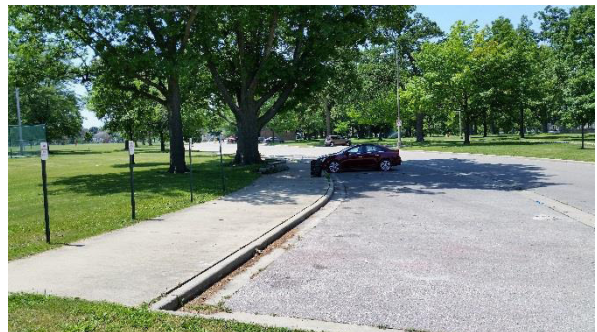
Faded parking striping
