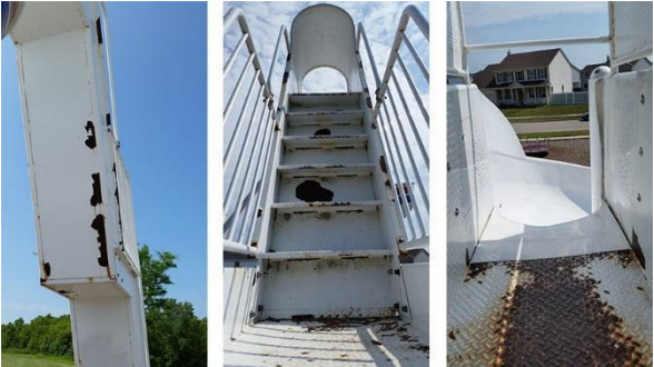
Metal slide in poor condition
