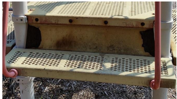
Play structure in poor condition
