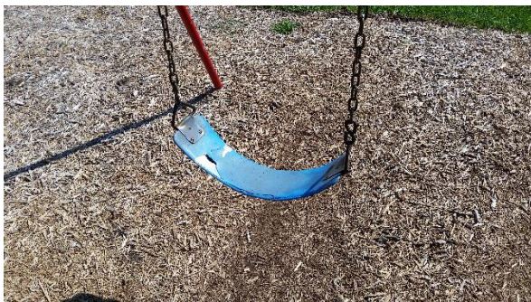
Belt swing seats are worn
