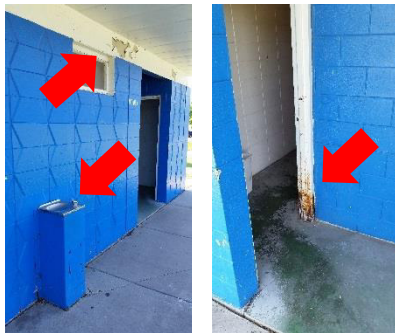
Restroom building issues
