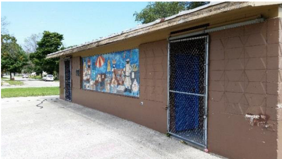
Restroom building is aging
