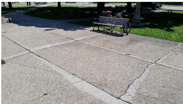
Concrete is cracking
