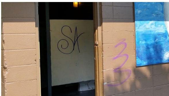
Graffiti at restroom building
