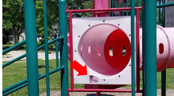
Play structure damage
