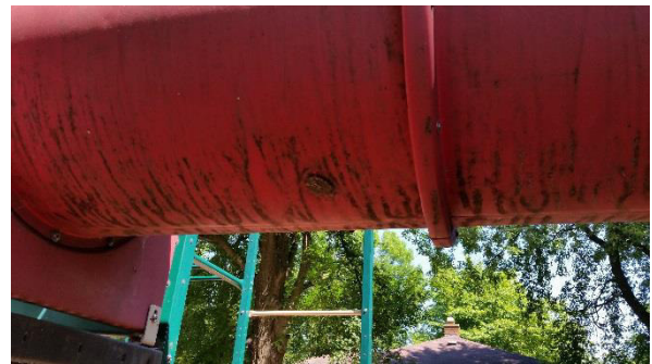
Play structure tube in poor condition
