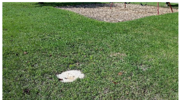
Concrete pad with exposed pegs (Trip hazard)
