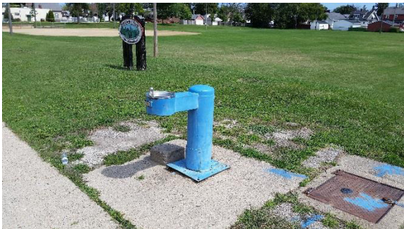
Drinking fountain is aging
