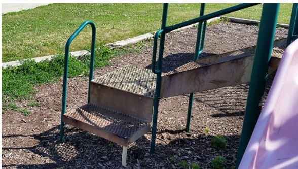
Play structure in poor condition
