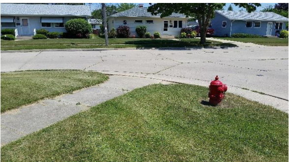
No curb ramp at walk to flagpole
