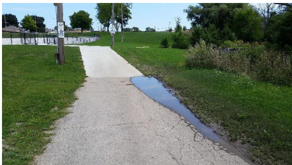
Path drainage issue
