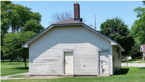
Building in poor condition
