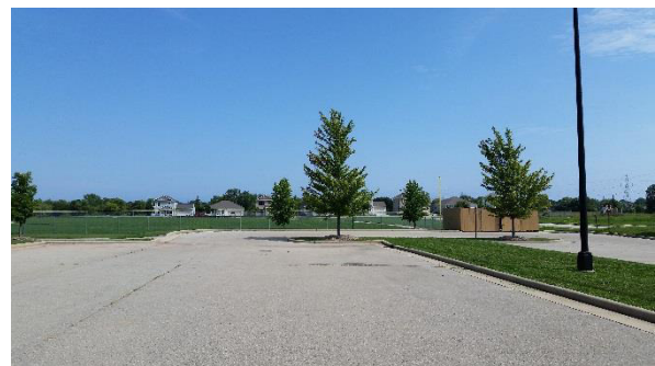
Faded parking lot striping
