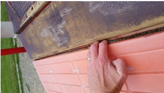
Pinch point on play structure bridge
