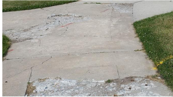
Path in poor condition
