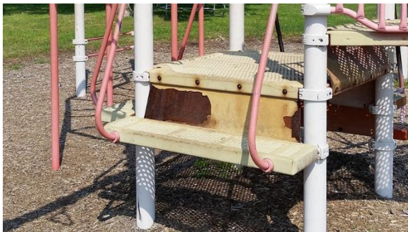
Play structure in poor condition
