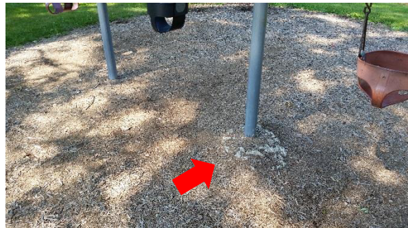
Concrete footing in fall zone of swings
