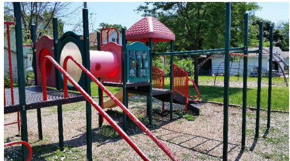
Play structure in poor condition
